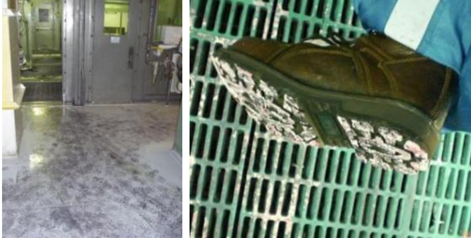
Paint Overspray and Paint Tracking Damage
